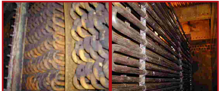
Complete re-tubing of exhaust gas boiler (economiser) with partial renewal of casing plate.
